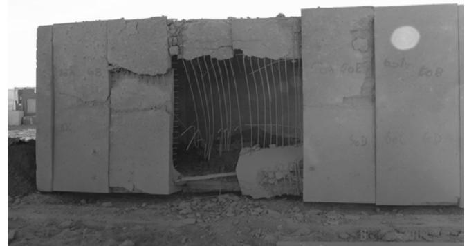
Figure 10: Breaching failure due to a close-in explosion of 6000kg TNT equivalent
